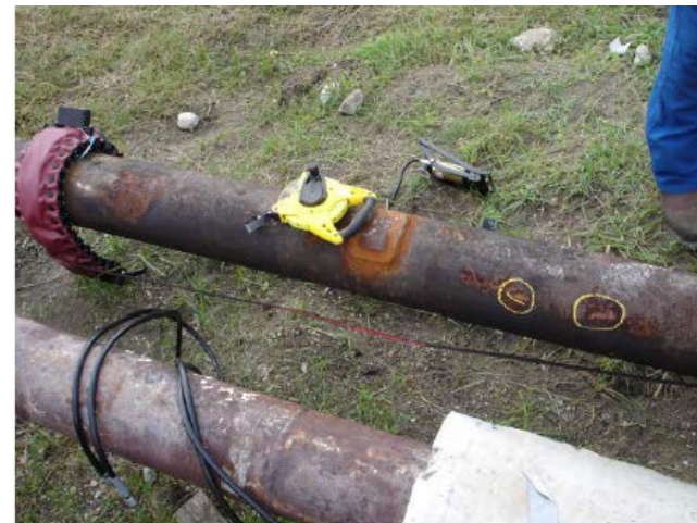
TL-01 Pitting - .120" - .140" deep
