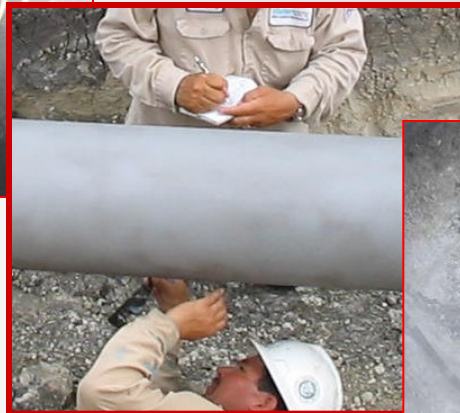
Mark Area for Repair
